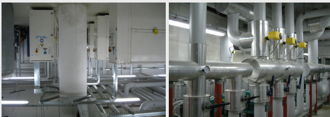
Centro Meridiana – 4P system heat pump and fuel headers
